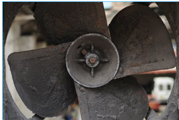
Figure 9: A dirty ventilation fan.
