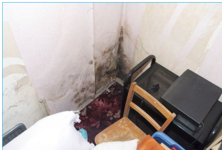
Figure 12: Mould growth and dampness.
