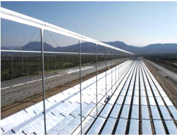
Figure 11 - Reflectors and receiver for a Linear Fresnel power station [8]
