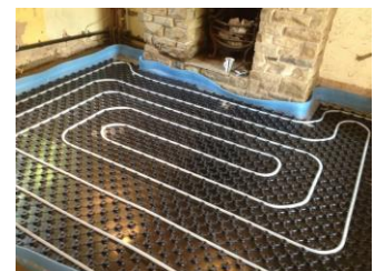
Figure 5 – Under Floor Heating
