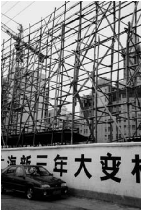
A residential area in central Shanghai in the process of being demolished. (Photo by Zhang Zhen)
